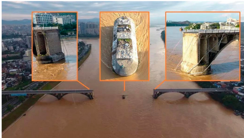
Figure 7. Broken column and bridge body on both sides of the column after collapse [Picture source: https://new.qq.com/omn/20190614/20190614A0E3YB.html ].
