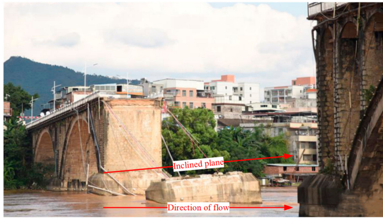
Figure 9. Inclination of the foundation of Pier 2.
